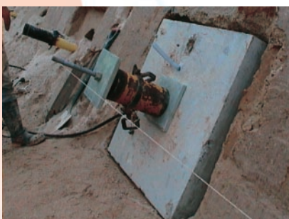
(left) screw piles were tensioned against concrete plates set into the embankment
