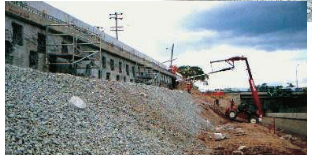
(Above) Screw pile being installed through penetrations cut in the shotcrete wall
